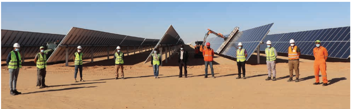
Solar panels installed at the Benban Solar Park, Egypt
